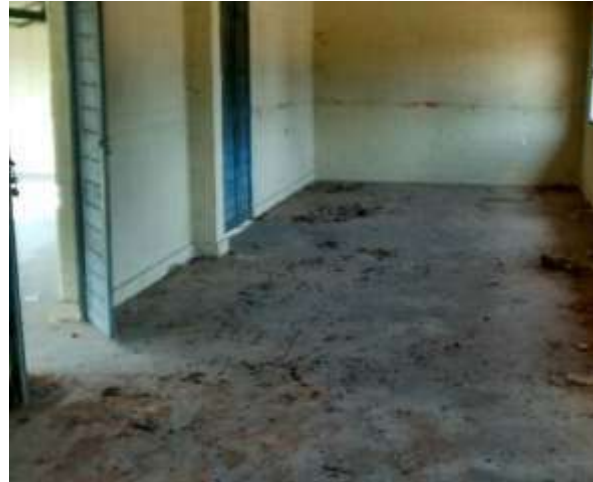
Community Hall Requiring Renovation, Kuthambakkam
