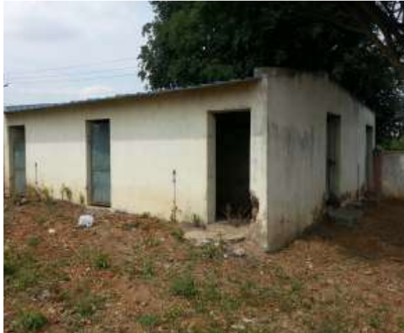
Restrooms Requiring Renovation: Melakotayur School
